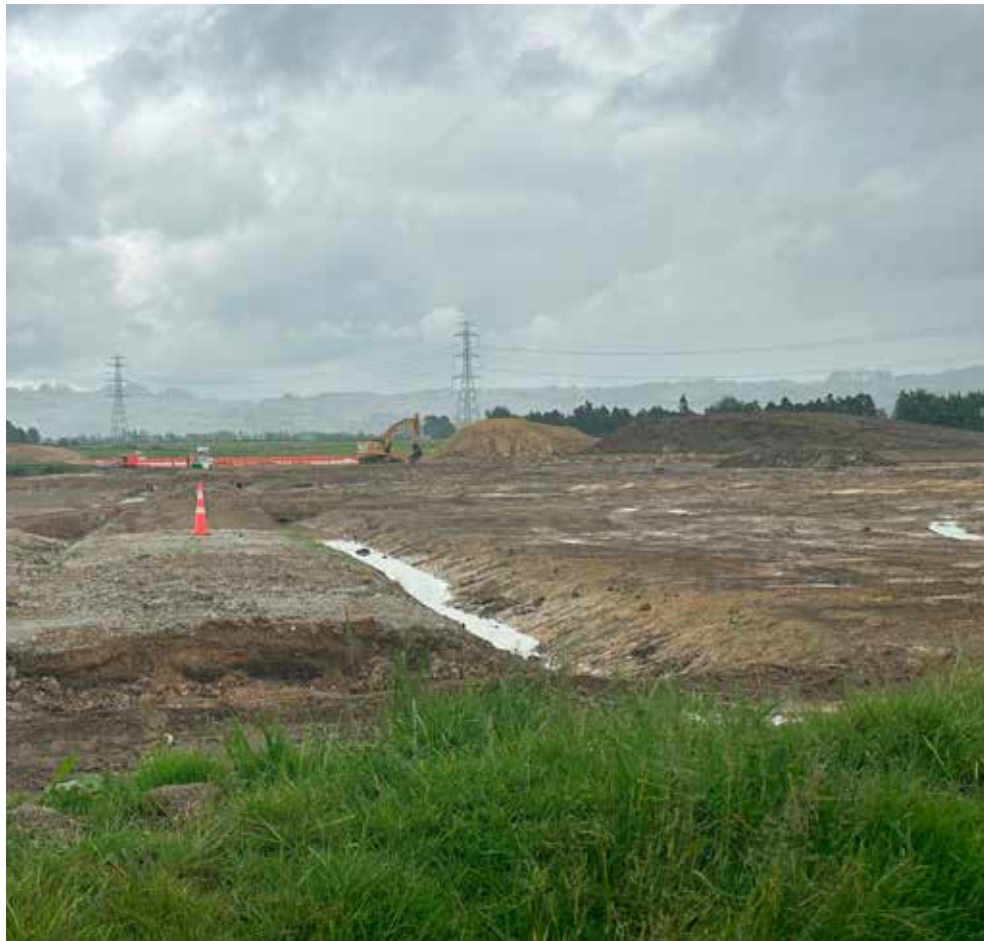
Earthworks are under way at Conmara Estate’s site on the southern side of Papakura Clevedon Road.
