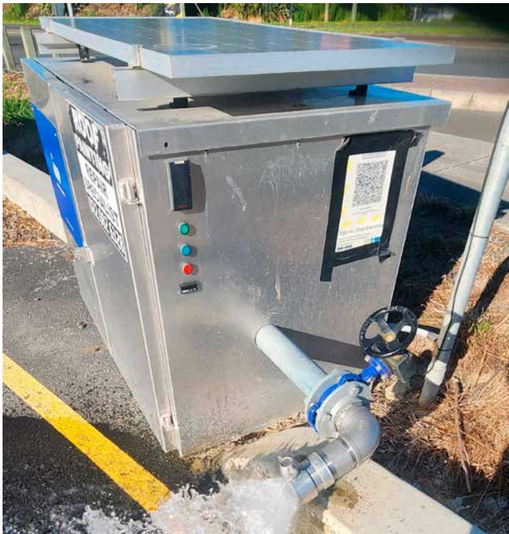
Coastal Purewater's hydrant delivers clean, clear water from an aquifer 275m below ground.
