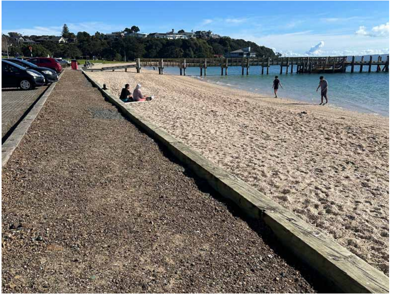
Maraetai's existing seawall has not fared well under the onslaught of storms and king tides.
